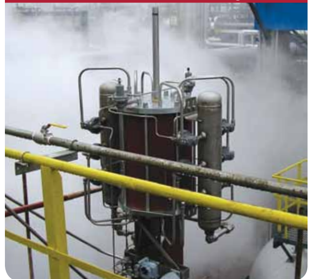
SVI II AP on steam conditioning valve
